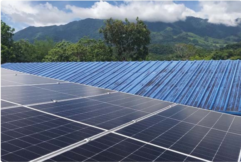
Solar panels installed at the ChocoAmazonic cooperative’s chocolate production plant in Caquetá, Colombia
